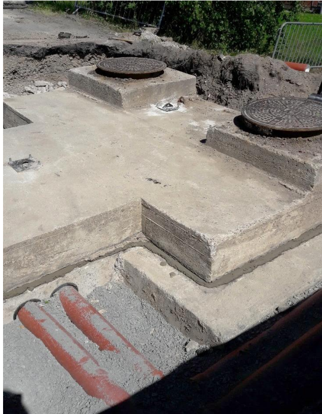
Figure 1. Covered DH chamber seen from above ground (Vattenfall, n.d.b).
